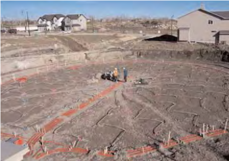
Seasonal Storage Borehole Field, Drake Landing.
